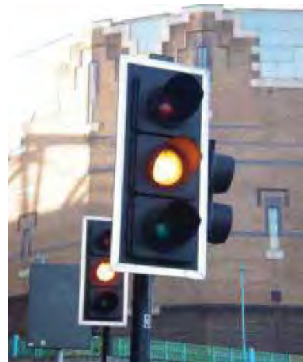
Traffic signals, image courtesy of Atkins
