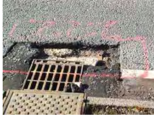
Damage to ironworks, image courtesy of Atkins
